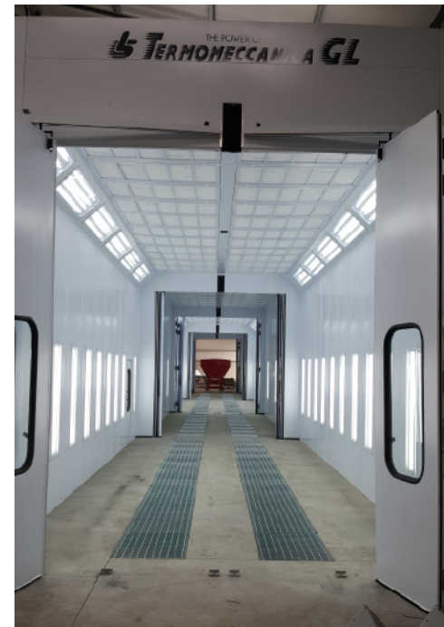
Spreader entering paint facility
