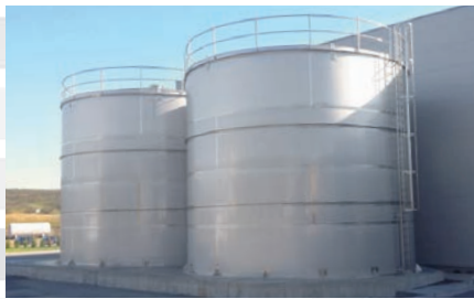
External free-standing tanks with capacity of up to 1 million liters
