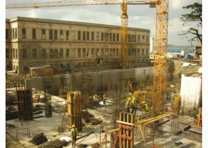
FOUR SEASONS HOTEL İSTANBUL, TURKEY Client: ASTAY GAYRİMENKUL İNŞAAT YATIRIM ve TURİZM A.Ş.
