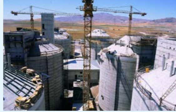
All Civil Works for Digester Tower (8pcs) and Boiler House and Service Tower by Mr. Veli Balkır Gürpınar.
