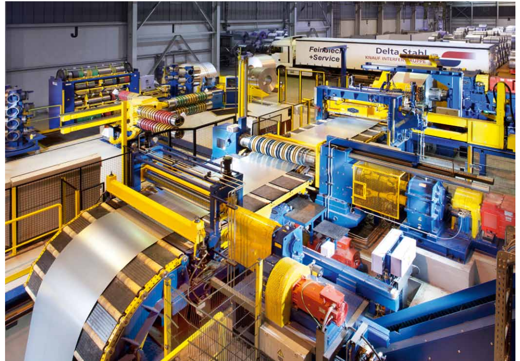
Slitting line in a steel service centre
