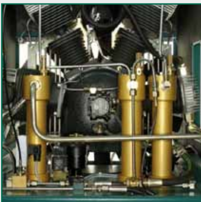
Water separators after each stage
