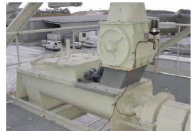
Mineral industry: lime factory: lubrication of 4 screw drive bearings.
