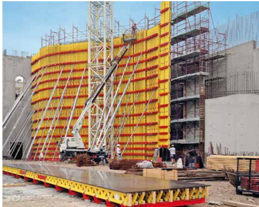
14 m high VARIO elements in a polygonal arrangement. Large-sized FinPly Maxi formlining sheets ensure excellent concrete surfaces.
