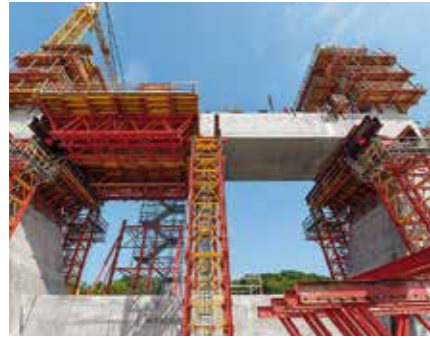
Heavy-Duty Shoring Towers and Truss Girders from the VARIOKIT Engineering Construction Kit provided a solid basis for forming the cross beams at the level of the road surfaces.
