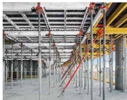
For the two flanking office towers, SKYDECK was supplemented at the slab edges with slab tables.
