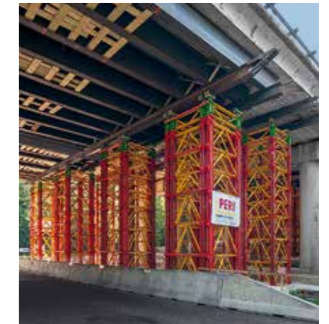
Concentrated: with the help of additional legs, the load-bearing capacity was individually adapted to accommodate the increased load from the carriageway bridging.
