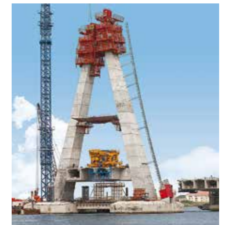
For the construction of this 90 m high pylon, the RCS and ACS climbing systems were combined.
