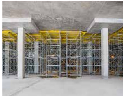
PERI UP shoring towers support the MULTIFLEX Girder Slab Formwork in order to efficiently construct the cast in-situ slab at a height of almost 8 m.
