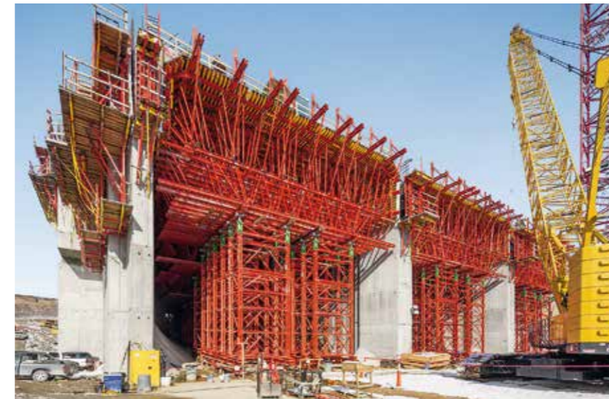
A customized unit and VARIOKIT heavy-duty shoring towers safely transfer the high loads of this over 4.00 m thick power station slab.
