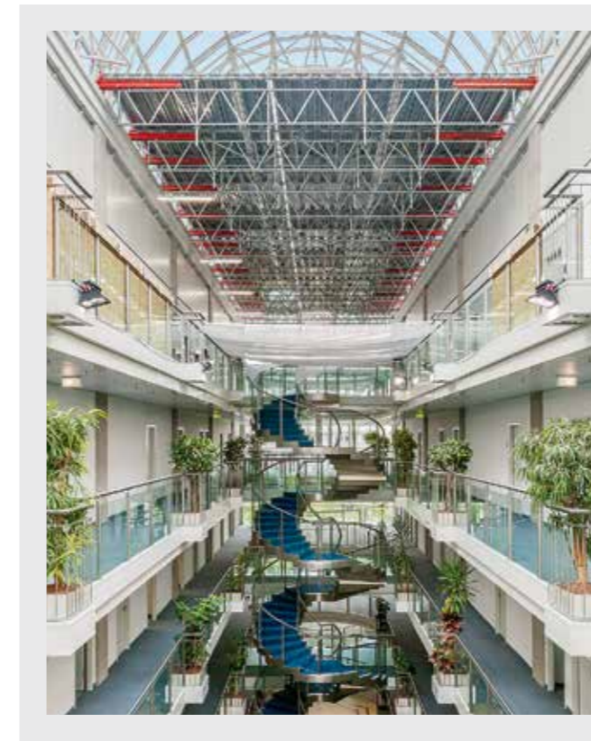
Platform and roof on the basis of the PERI UP scaffolding system allow safe and uninterrupted renovation work on the arched glass roof. The scaffold simultaneously protects the public areas positioned below.
