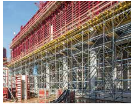
The planning and supply of formwork and scaffolding from one source created a synergy effect for the site management team.
