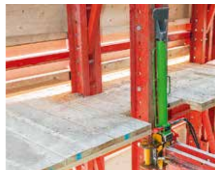
Mobile climbing units lifted the rail-guided RCS Climbing Protection Panel from storey to storey.
