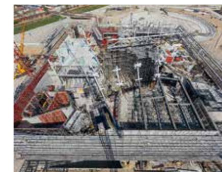
PERI Italy planned and delivered almost 800 m 2 of special steel formwork as well as 2,000 m 2 TRIO and 2,500 m 2 SKYDECK in a very short time.
