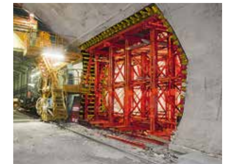
This tunnel formwork carriage on the basis of the VARIOKIT modular system is used for constructing the accessible cross passage between two tunnel tubes.
