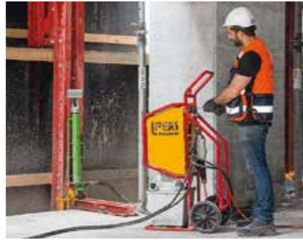
The RCS Climbing Protection Panel units climbed crane-independently with the help of mobile self-climbing devices to the next floor each time.
