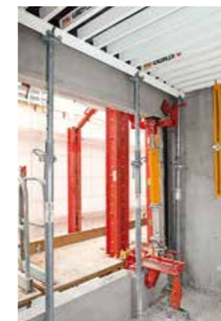
Several RCS Climbing Rails were anchored on the parapets and additionally fixed to the slab.
