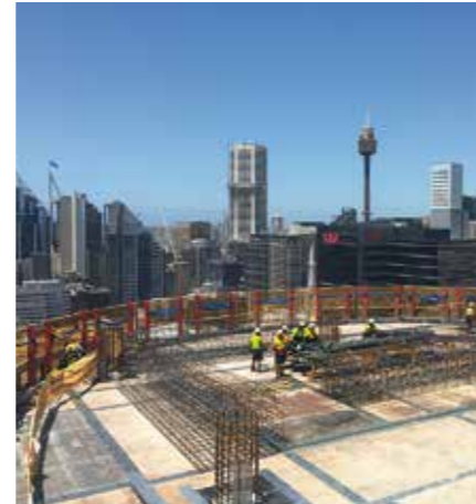
Over 700 linear metres of PERI LPS enclosure secured and accelerated construction work on the three high-rise towers.
