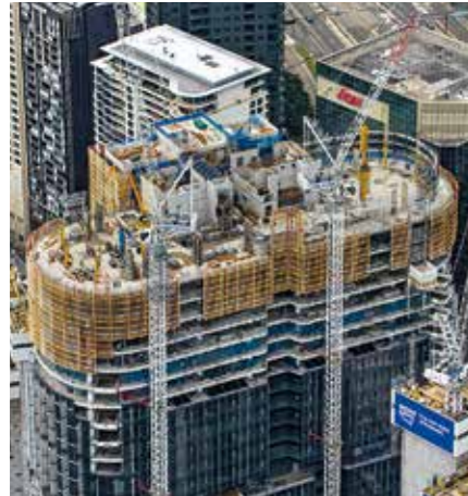
The protection panel units up to 18.50 m high climbed by means of mobile climbing hydraulics to the next floor without requiring a crane.
