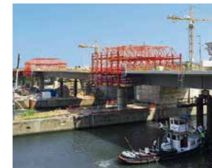
This lock bridge is being constructed with 2 VARIOKIT Composite Formwork Carriages in 13 casting segments using the back-step construction method.
