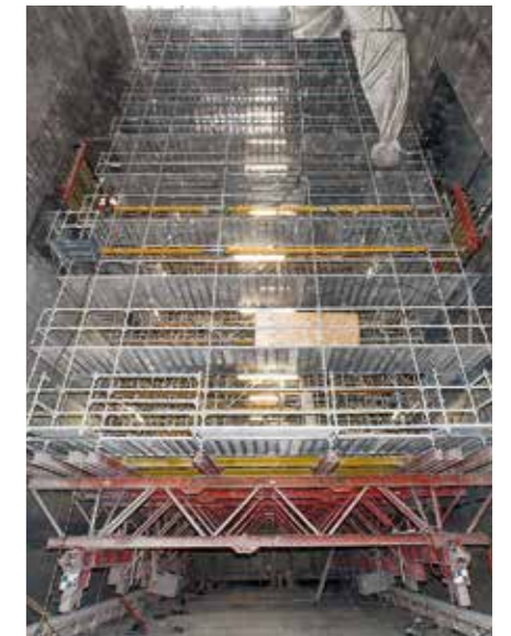
VARIOKIT components form the basis for the mobile, up to 90 t scaffold bracket for sand blasting and forming operations during a refurbishment project.
