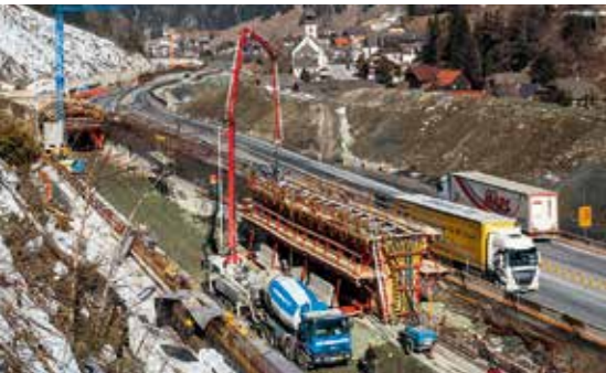
With help of the VARIOKIT Tunnel Formwork solution, 25 m long sections of the tunnel arch could be concreted in regular 4-day cycles.
