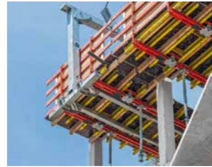
The VARIODECK Edge Tables were moved as large-sized units including guardrails with the help of the PERI Transportation Fork.
