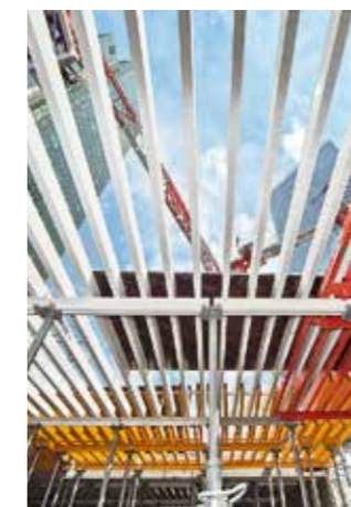
Construction of the floor slabs was carried out with help of GRIDFLEX Girder Grid Slab Formwork system.
