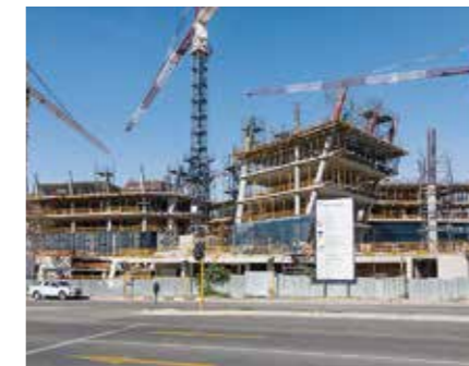
The administration building is characterized by obliquely-arranged building structure and cantilevered slabs.
