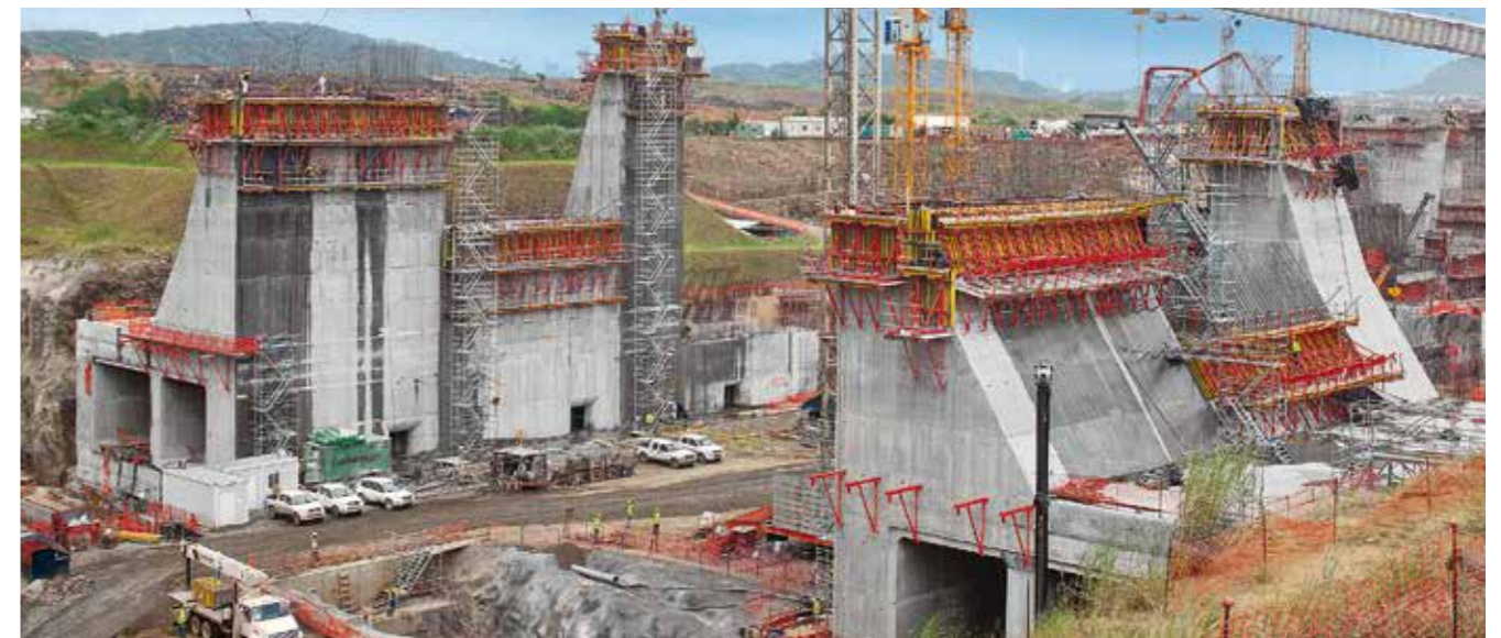
Use of SCS Climbing Formwork for the construction of the new locks in the Panama Canal.
