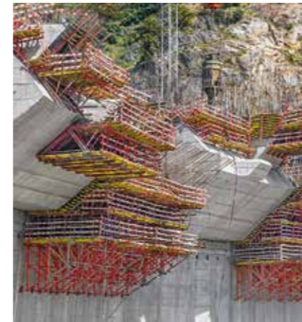
The SCS 190 Climbing System in combination with VARIO GT 24 Girder Wall Formwork for a double-curved dam wall.
