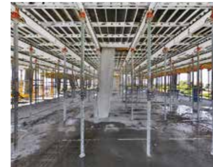
The slabs were formed with the help of the SKYDECK system in rapid cycle sequences.
