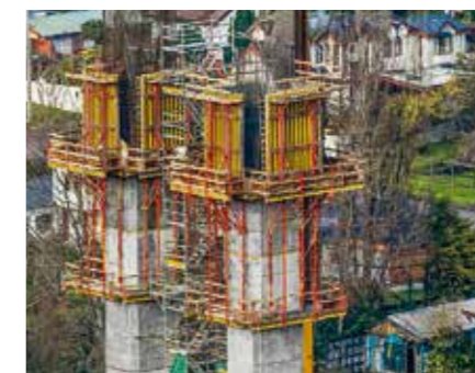
The CB Climbing System and VARIO GT 24 Girder Wall Formwork formed crane-movable climbing formwork units for the up to 40 m high double piers.
