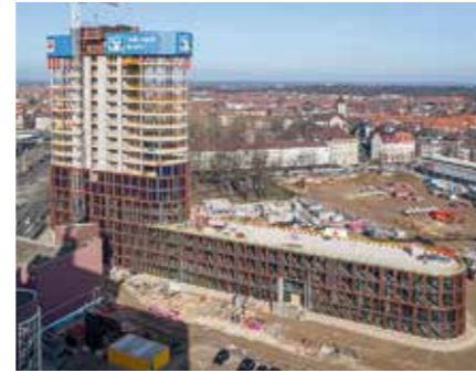
The 70 m high-rise building and the 120 m long base construction were completed in a concrete shell realization phase of only 10 months.
