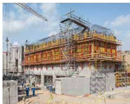
The PERI system application was matched to suit the massive reinforced concrete components with slab thicknesses up to 2.50 m and large supporting heights of up to 10 m.
