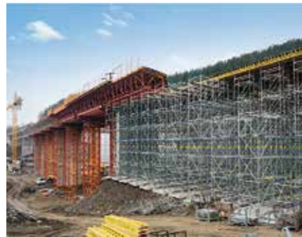
Cost-effective: the PERI bridge formwork concept was based on rentable modular construction systems with standardized components.
