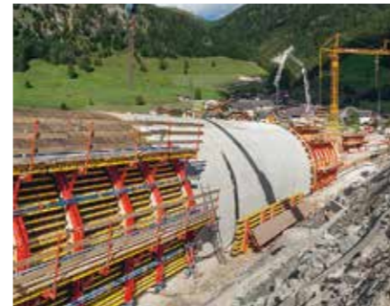
The external formwork for the tunnel arch was moved as large-sized units with the crane.
