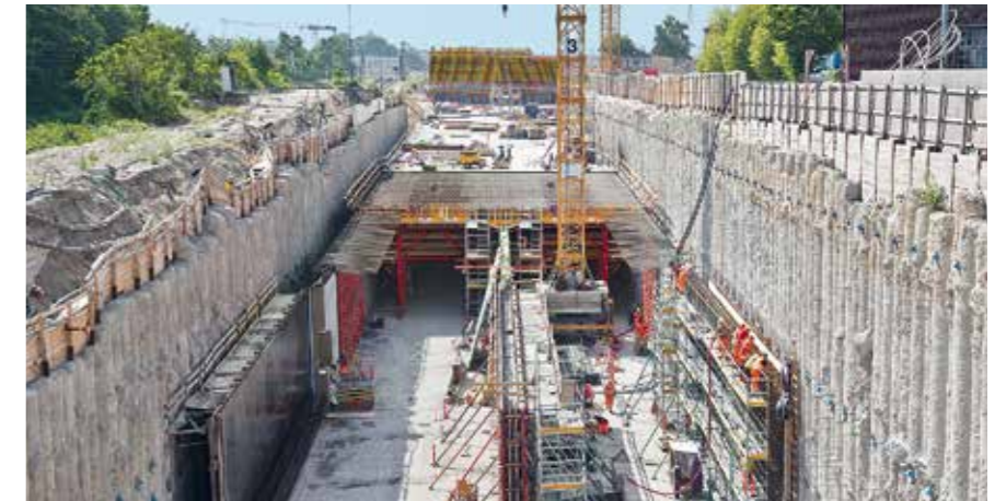
The “Nordhavnsvej – Vej- og Tunnelentreprise” major infrastructure project connects the North Harbour in Copenhagen with the Helsingør motorway. The 620 m long tunnel route runs through a very densely built-up inner city area and also crosses a busy railway line.
