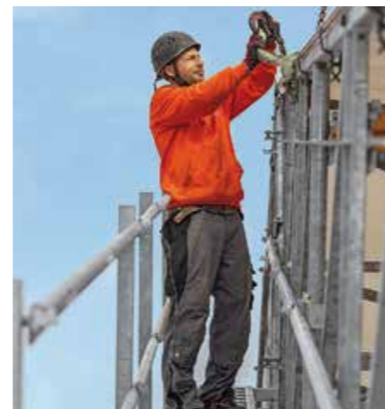
Walkways along the girders ensure safe access during the assembly of the individual segments.
