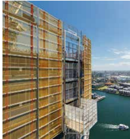
Two RCS Landing Platforms were integrated into the LPS enclosure on each tower and supplemented with additional protective meshes.
