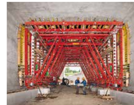
Depending on requirements, components of other PERI systems supplement the VARIOKIT solution; with this formwork carriage, for example, HD 200 Heavy-Duty Props.
