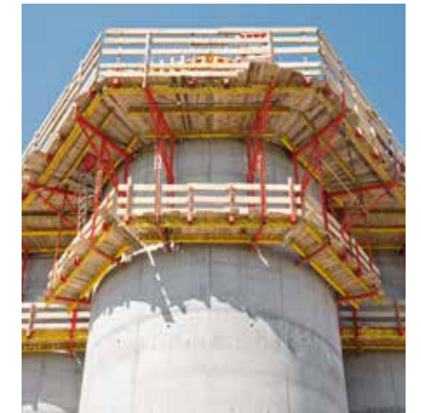
Climbing formwork solution with CB Climbing Platforms and dimensionally-accurate rounded VARIO GT 24 Wall Formwork.
