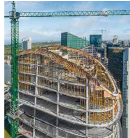
The edge beam construction for the tower finish placed very high requirements on construction operations.
