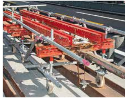
The VARIOKIT carriage for suspending the PERI UP suspended scaffold by means of DW 15 tie rods could be moved within the existing crash barriers.
