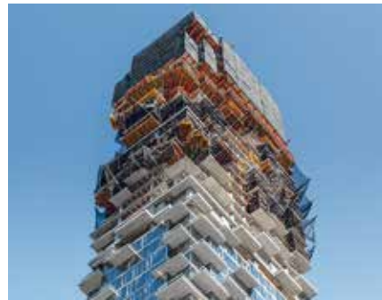
Offset-arranged floors and countless cantilevered balconies required a detailed formwork and enclosure concept.
