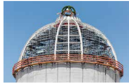
The 70 m high cupola roof towers above the 180 m long city palace which, behind its historical Baroque appearance, serves as a modern-style Humboldt Forum for exhibitions.
