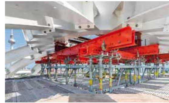
The PERI UP and VARIOKIT Modular Construction Systems ideally complemented each other for the temporary transfer of loads from the steel cupola.
