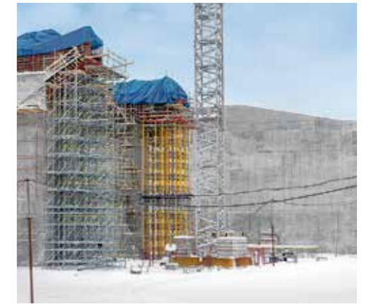
The massive reinforced concrete piers widen out in the head section. MULTIPROP and PERI UP reliably transferred the high loads from great heights into the ground.
