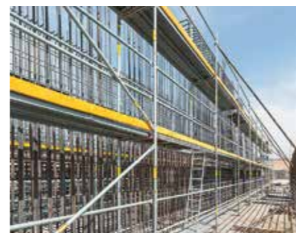
PERI UP Frame Scaffolding is being used for the time-consuming reinforcement work.
