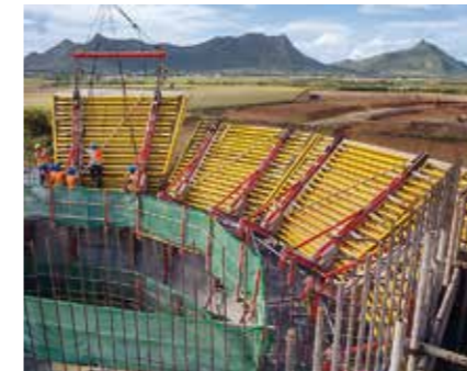
Special suspension points ensured that the formwork elements could easily be lifted into the respective final position with the crane.
