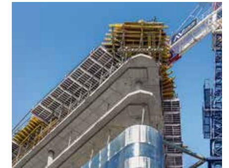
On the building corners, individually planned slab tables supplemented the cantilevered-mounted SKYDECK edge solution.
