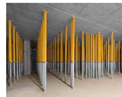
Lightweight aluminium MULTIPROP Slab Props were used to provide support over the height of several floors.
