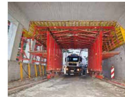
With this slab formwork carriage, a 3.00 m wide and 4.50 m high drive-through opening ensured unobstructed site traffic operations.
