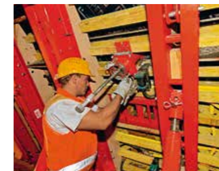
Concrete pump connections and vibrators are planned and supplied according to needs and requirements.
