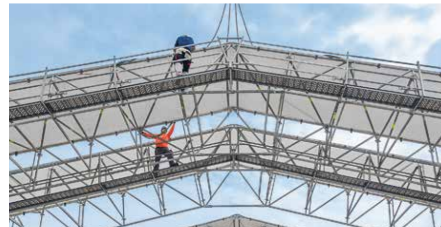
The roof segments can be pre-assembled on the ground, subsequently they are lifted by crane to their final position.
