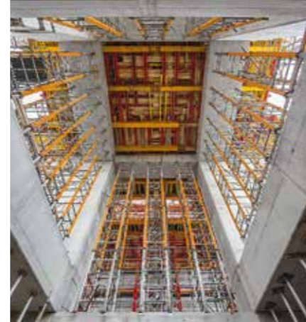
Modular supporting systems made it possible to easily adapt to the complex building structure.
