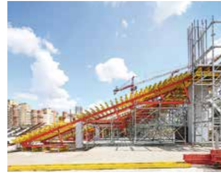
The two modular construction systems, VARIOKIT and PERI UP, formed shape-generating shoring for realizing the inclined grandstand stringers.
