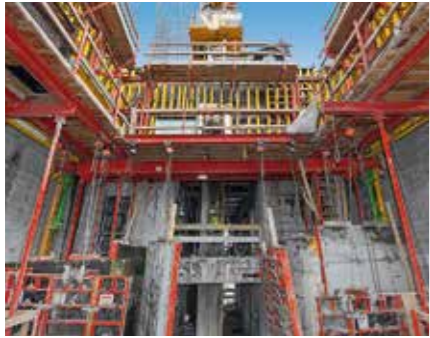
The self-climbing ACS P Platform variant was adapted to suit the central 8 m x 10 m core ground plan while suspended DOMINO elements served for subsequently constructing the intermediate walls.
