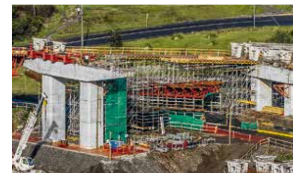
Also for bridging the main road situated in the ramp area of Chamiza Viaduct, PERI UP and VARIOKIT supplemented each other perfectly.
