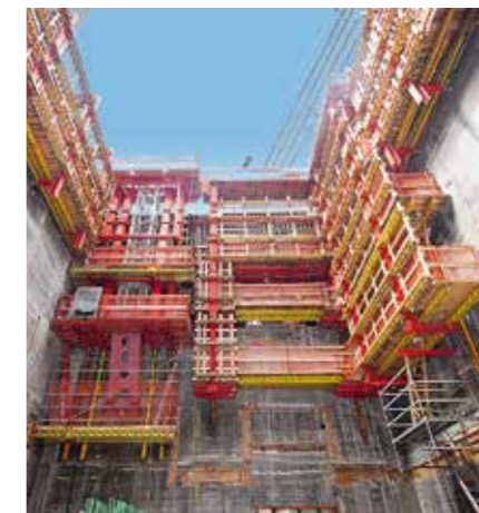
With the ACS self-climbing technology, the concrete placing boom and suspended stair towers can also be moved upwards with any crane assistance.
