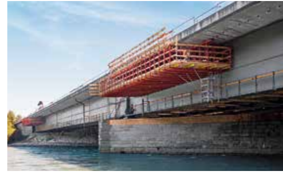
The refurbishment of the 185 m long Inntal Bridge was carried out by two complementary PERI modular construction systems – to a large extent without restricting road traffic.
