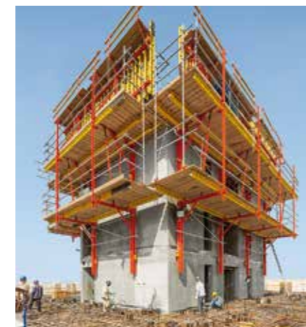
Contractor Azmeel Contracting & Construction Corporation Field Service PERI Saudi Arabia Ltd., Jeddah
