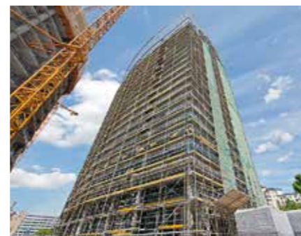
PERI UP Facade Scaffolding allowed fast and safe execution of all reworking operations
