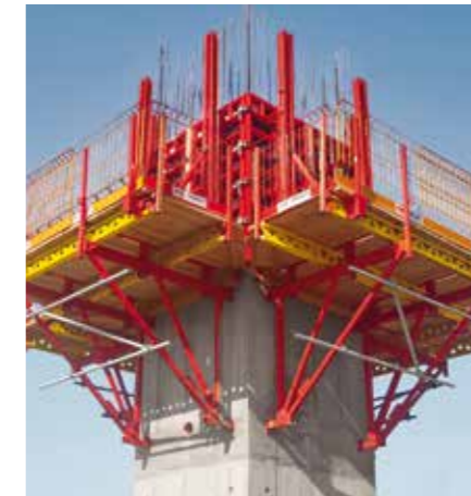
Use of the CB 240 Climbing Formwork with TRIO Wall Formwork for a 27 m high tower building. The BR Shaft Platform supports the shaft internal formwork.
