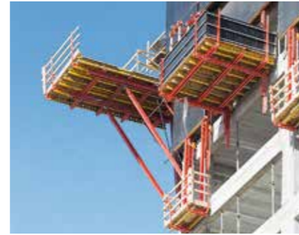
For forming the oblique-angled building corners – due to the facade inclinations – specially designed corner platforms were used which were based on system equipment.
