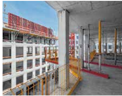
PROKIT provided gap-free enclosure of the building shell slab edges, including the transition area to the cantilevered-mounted RCS MP Landing Platform.
