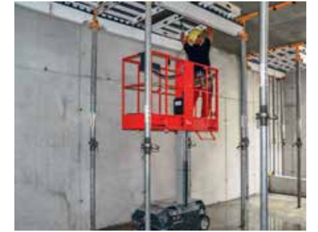
The lifting platform allows safe shuttering and striking operations. It can also be used for reworking tasks or dismantling the shoring construction.
