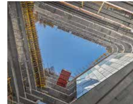
In spite of the complex building geometry, work could be carried out to a large extent with system formwork.
