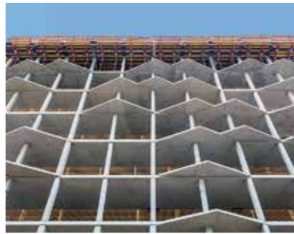
VARIODECK and PROKIT guaranteed a high level of safety during construction of the residential towers complete with triangular oriels.
